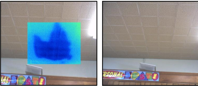
Thermal Image (left) shows extensively water saturated ceiling, while there is no visible evidence of water damage (right).
